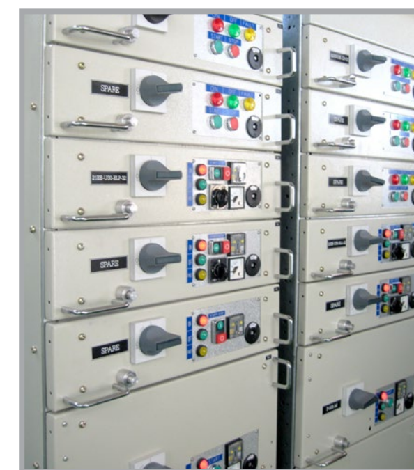
Low Voltage Withdrawable Panels
