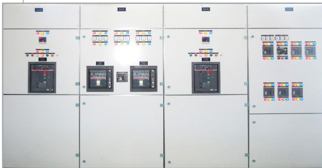
Low Voltage Distribution Panels
