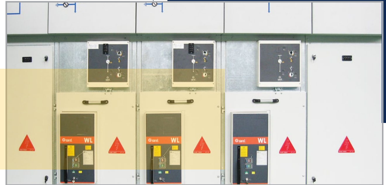
Medium Voltage Switchgears
