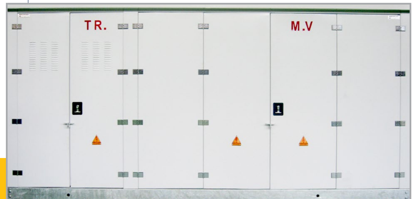
Medium Voltage Kiosk
